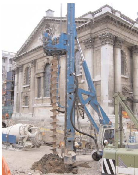
Above: concrete piling work begins. Right: recent view of the site looking towards Charing Cross.
